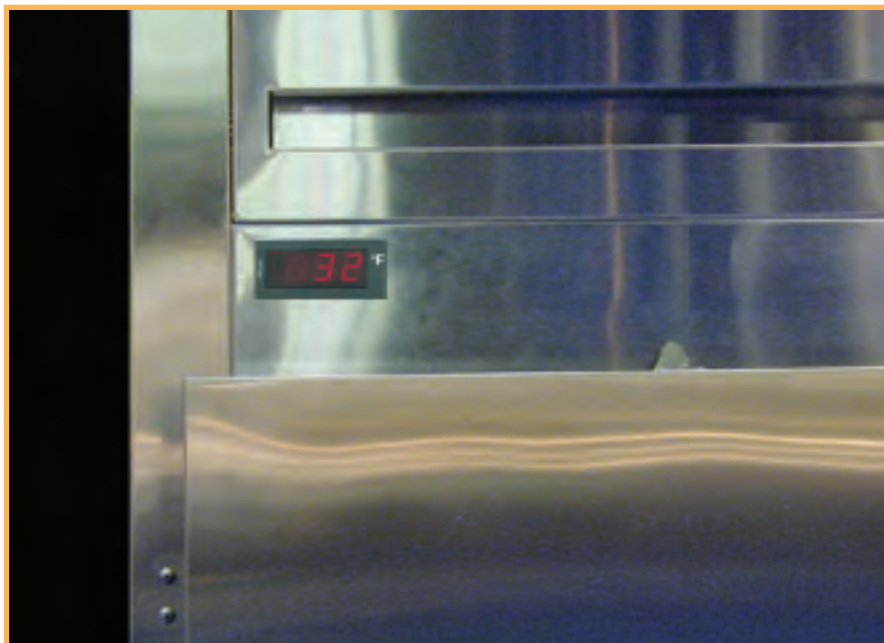
Reach-in Refrigeration / Freezers
